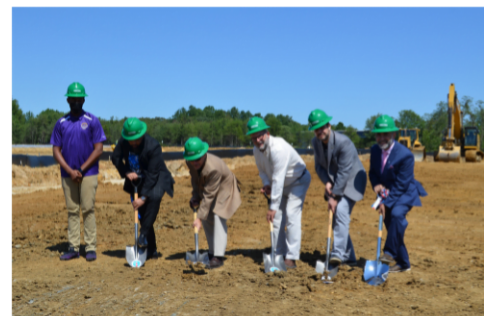
After having to reschedule due to inclement weather, the CLF & CMIT South Teams decided to make it happen. The groundbreaking ceremony for the CMIT South greenfield was a wonderful team cementing experience enjoyed by staff, family, community partners, and students!
